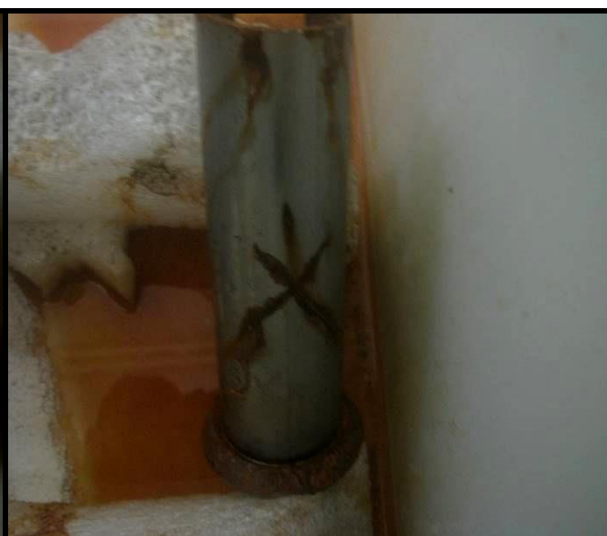
Photograph 26 showing the Sample 2 surface after 72 hours of continuous salt spray exposure.
