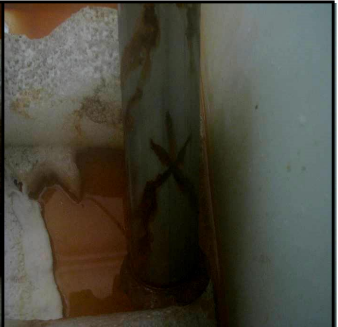
Photograph 30 showing the Sample 2 surface after 168 hours of continuous salt spray exposure.
