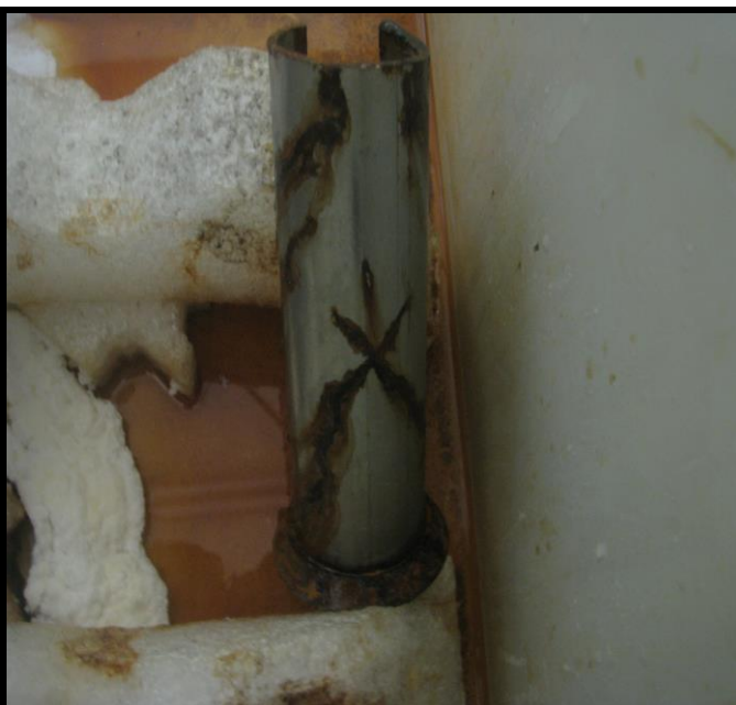
Photograph 32 showing the Sample 2 surface after 336 hours of continuous salt spray exposure.
