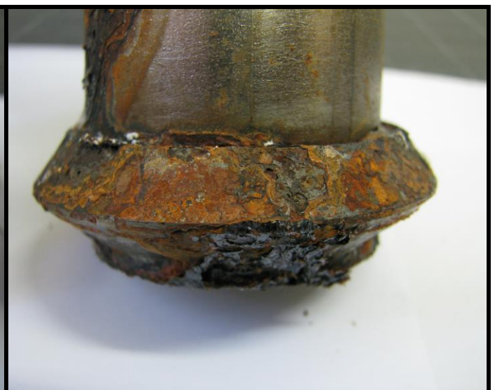
Photograph 16 showing the corrosion due to the run-off staining at the bottom section of Sample 2 after the 1000 hour exposure.
