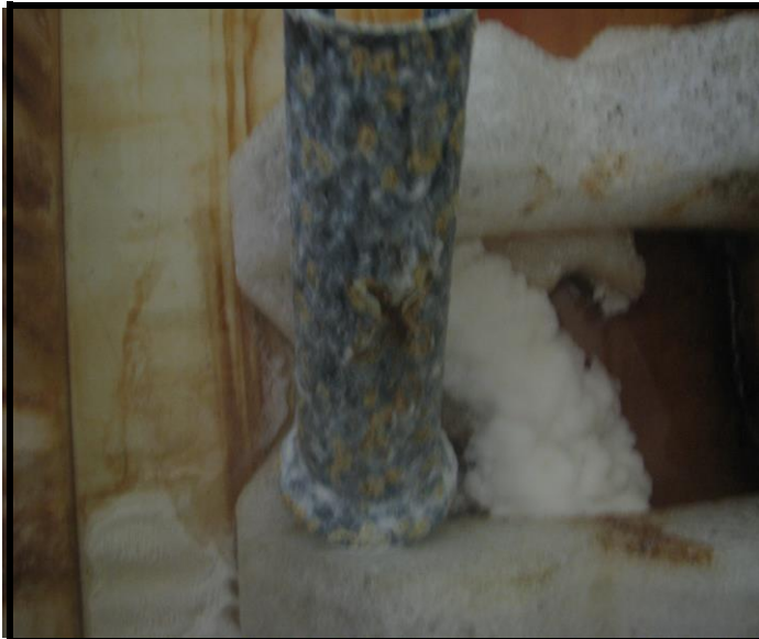
Photograph 35 showing the Sample 1 surface after 672 hours of continuous salt spray exposure.
